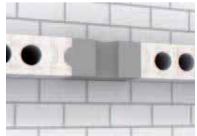
Porous concrete ceiling (possibly with cavities)
